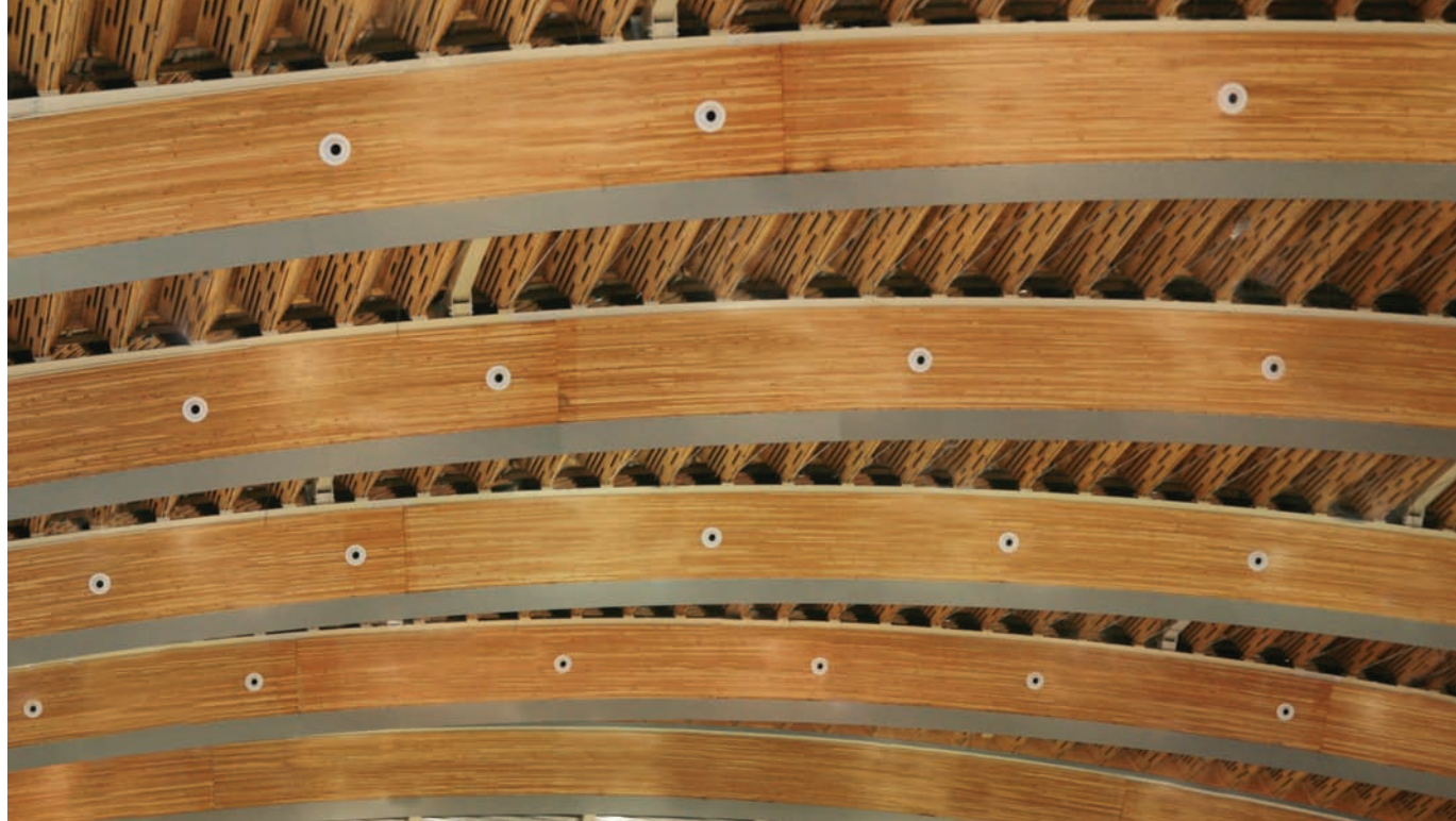
Ventilation system directional nozzles embedded in the glulam arches
